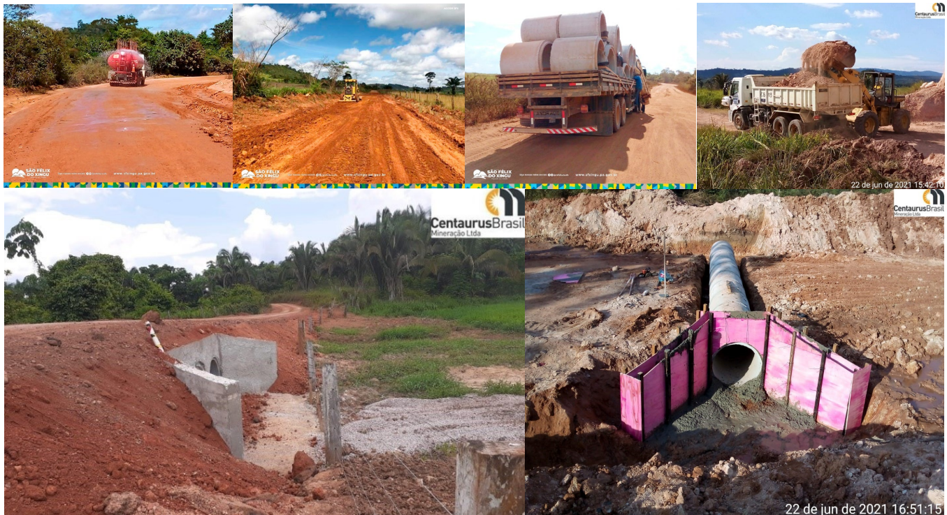
Figure 9 – Roadwork being undertaken under public private partnership with São Félix do Xingu Municipality
