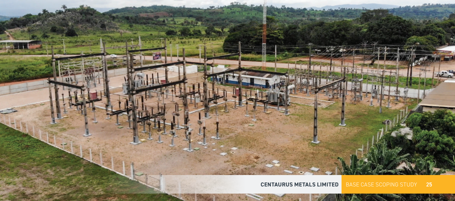
Figure 18 - 138kV National Grid connection at Tucumã
